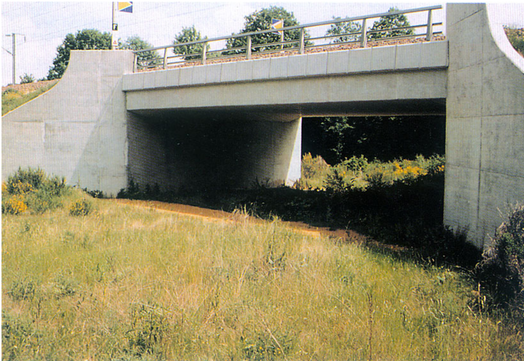
Figure 7.7 - Underpass under a high-speed railway line in France. (Photo by C.E.T.E. de l'Ouest)
