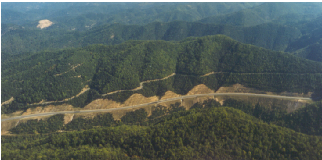
Figure 3.2 - Slope cuttings along a road in Spain. (Photo by Martí Pey/Minuartia Estudios Ambientals)
