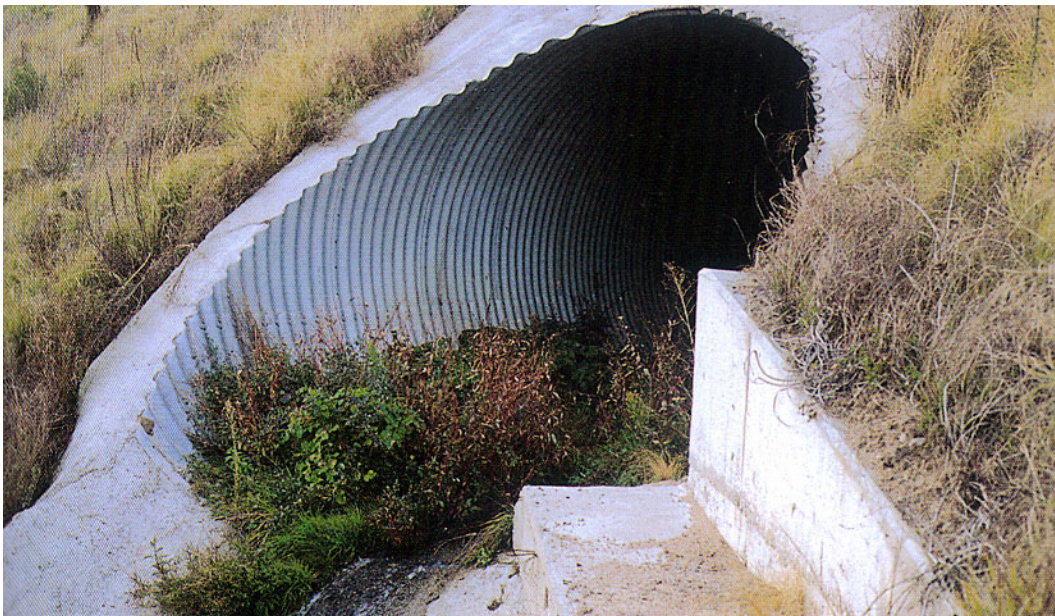
Figure 7.14 - A drainage culvert in Spain, used as a fauna passage. (Photo by Carme Rosell/Minuartia Estudi Ambientals)
