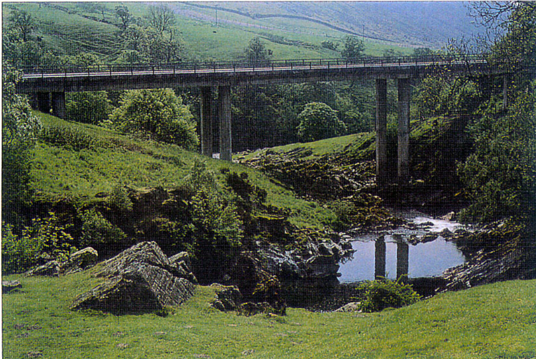
Figure 7.10 - A viaduct in England, leaving the natural landscape and vegetation intact. (Photo by Highways Agency, U.K.)
