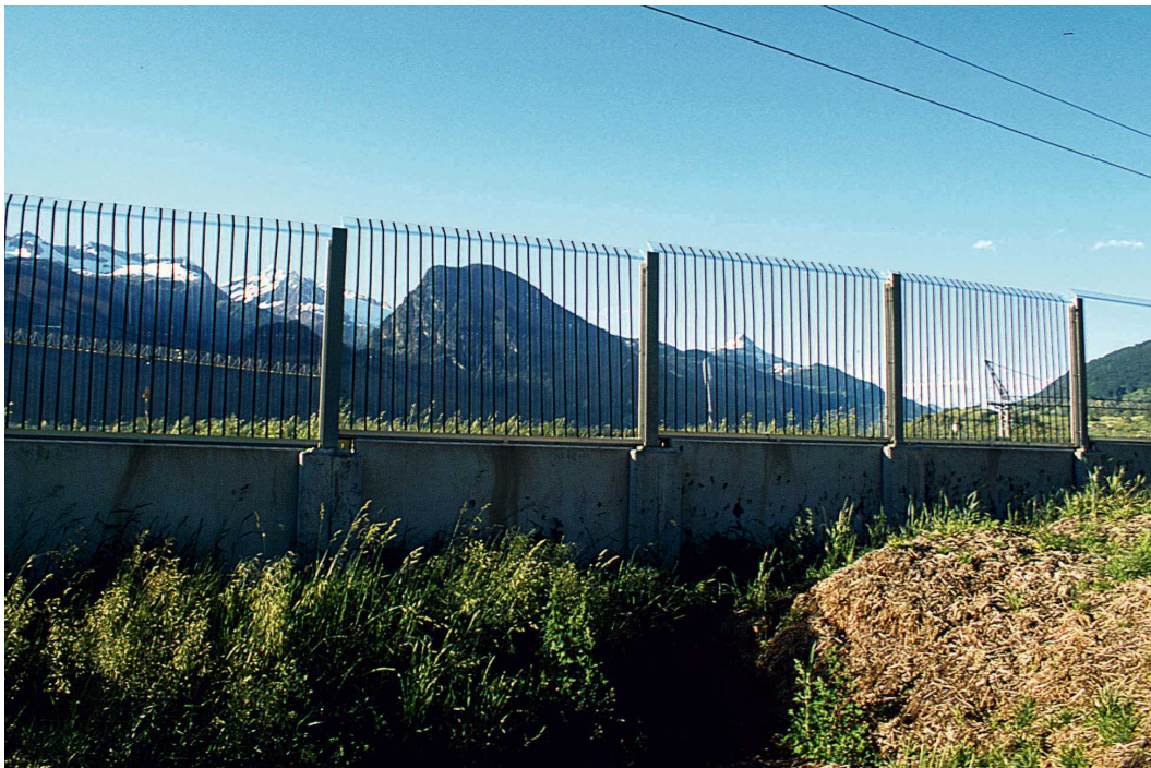
Figure 7.17 - A transparent noise barrier in Switzerland marked with stripes to reduce collisions of birds. (Photo by H. Schmid)
